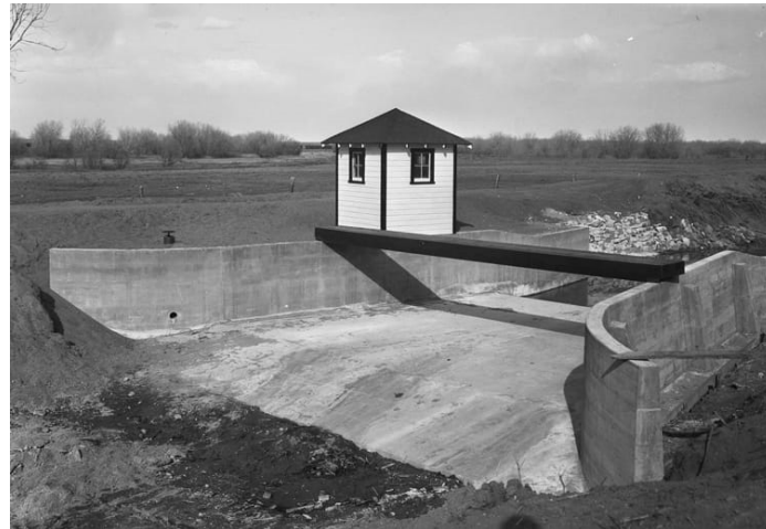
Figure 1. Parshall flume measuring structure, installed [2].
