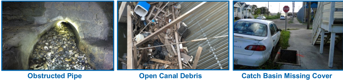
Figure 6: Collection System Issues
