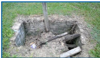
Collapsed Catch Basin
