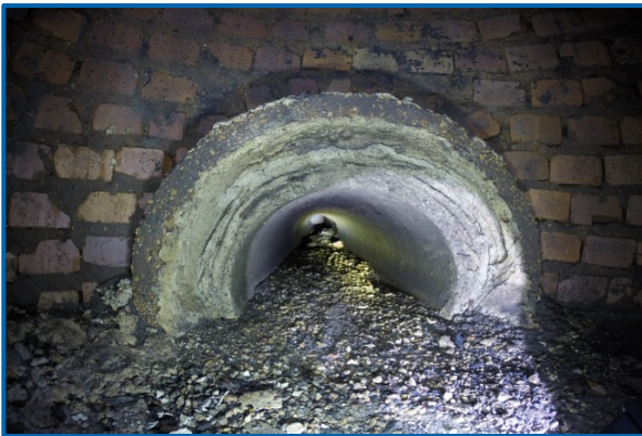
Pipes 27% Diminished Capacity
