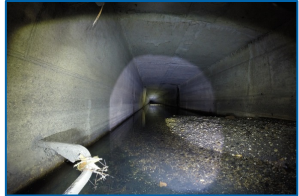
Box Canals 22% Diminished Capacity
