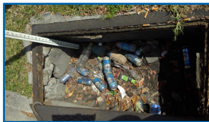
Catch Basin Debris
