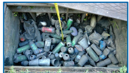
Catch Basin Debris
