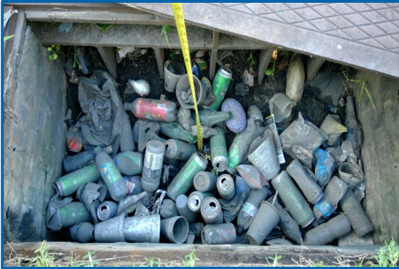
Catch Basins 16% Diminished Capacity
