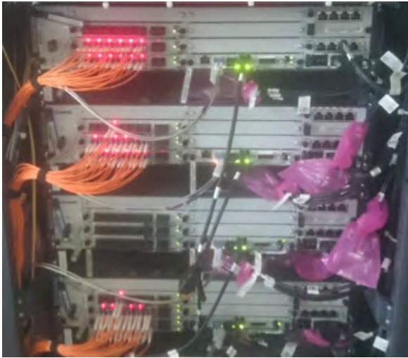
FIGURE 5. BBU pool used in TT central office location of C-RAN in Cekmekoy district of Istanbul.
