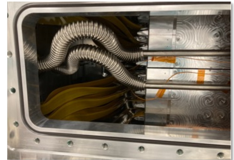
Deformed DSSC cooling pipes
