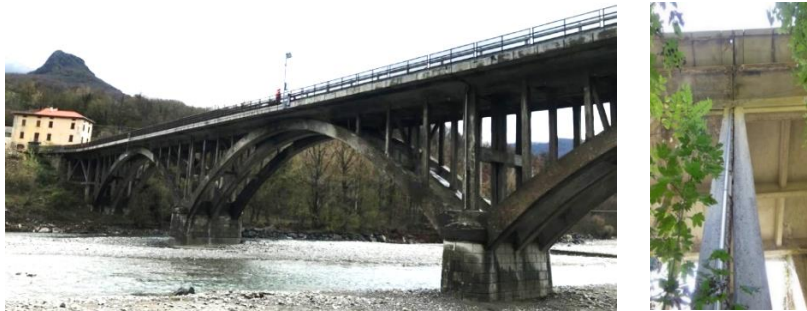
Fig. 1. Lamberti Bridge on the Ceno river (a); joint connecting two spans (b).
