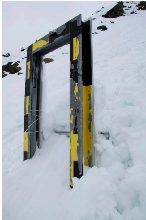
Figure 13. View of the obstacle after the event on 30 April 2014 (photo M. Maggioni on May 1). It is clearly visible that the plates are totally submerged in the snow and the large snow agglomerate against the structure.
