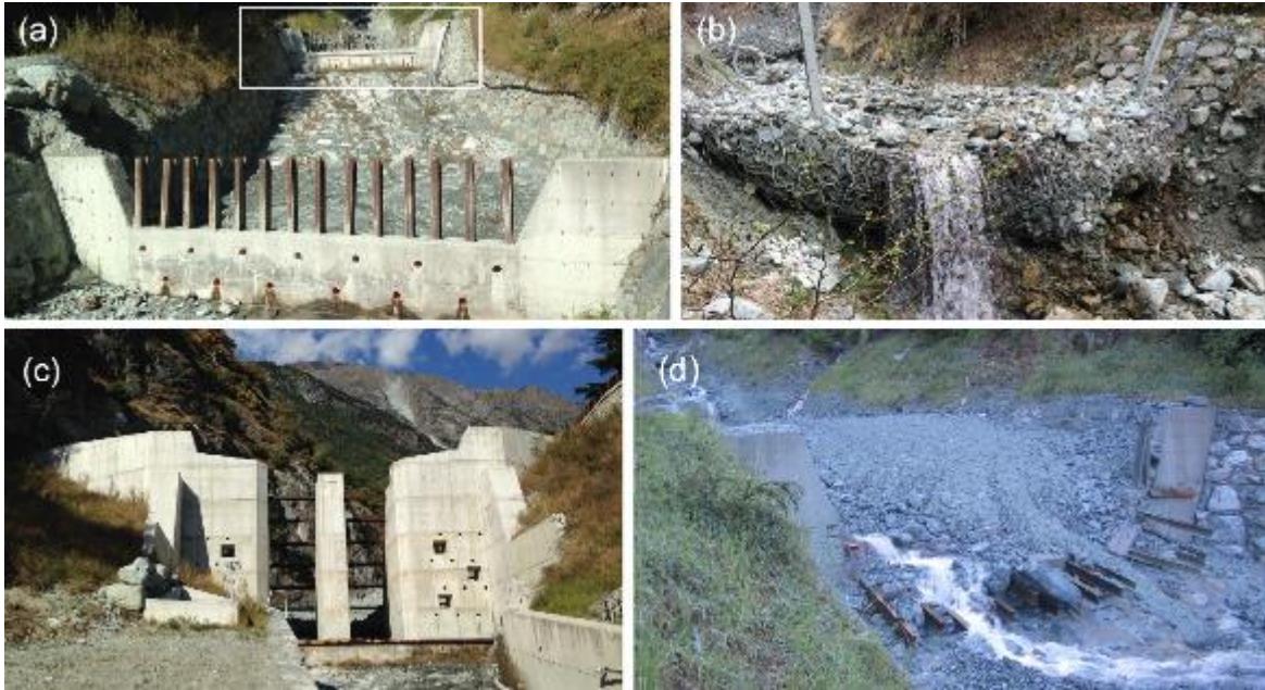
Fig. 2 The structural mitigation works along the Grand Valey torrent: (a) the two filter barriers at the Pèrriere hamlet; (b) the steel net barriers; (c) the slit-filter barrier at Tromen; (d) the barrier at Pèrriere (white rectangle in Fig. 2a) that collapsed in 2014. The position of each of these structures is indicated in Fig. 1 (photos courtesy of the Aosta Valley Autonomous Region).
