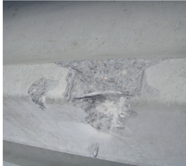
Figure 10 Damage of the protective concrete cover in the widened lower part of beam No. 6 from the Kapshagai side (The longitudinal smooth reinforcement is damaged)
