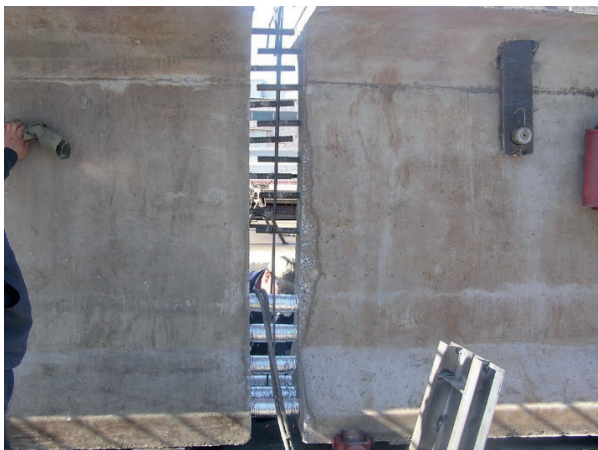
Figure 5 Joint zone No. 2 between the blocks before tensioning strands and concreting the joint (see Figure 1)
