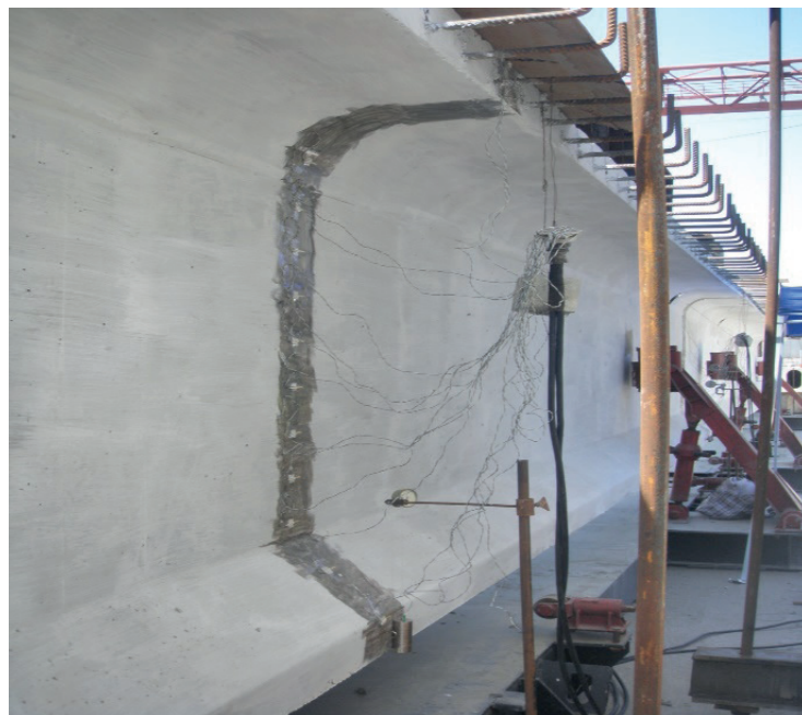
Figure 12 Fragment of a composite beam 42.0m long with installed strain gages and deflection meters in a beam with a monolithic joint
