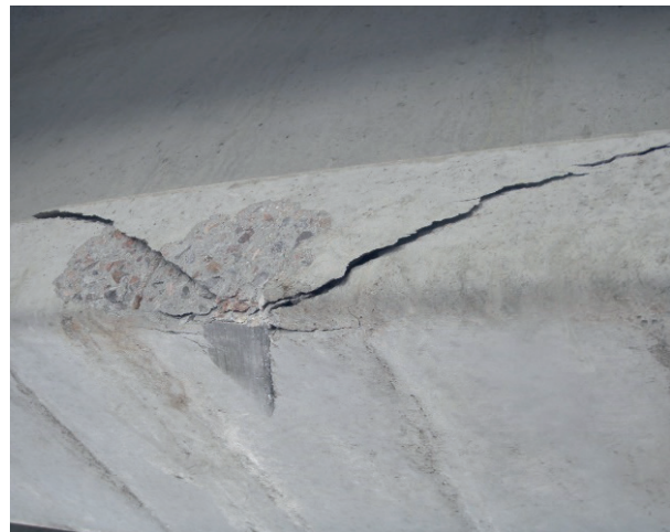
Figure 12 Destruction of the widened lower part of the beam No. 8 from the Kapshagai side
