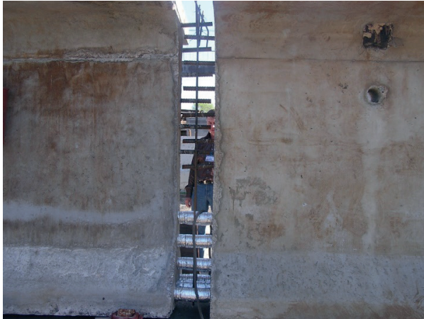
Figure 4 Joint zone No. 1 between the blocks before tensioning strands and concreting the joint (see Figure 1)
