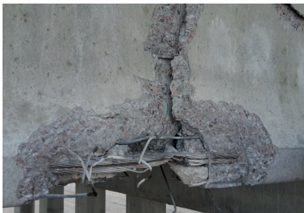
Figure 4 Fragment of destruction in beam No. 1 and damage with wire rupture of K-7 ropes from the Kapshagai side
