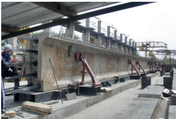
Figure 6 General view of the end block with tendons embedded in the ducts
