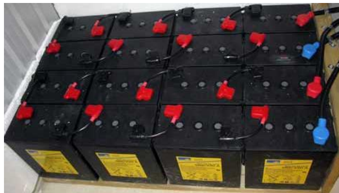
Figure 4. Battery system connection with 16 batteries.
