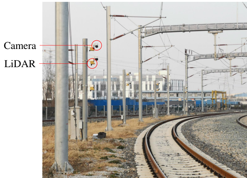
Figure 8. Railway monitoring equipment.
