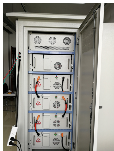
Figure 7. Basic information of LFP batteries on an experimental ESS.
