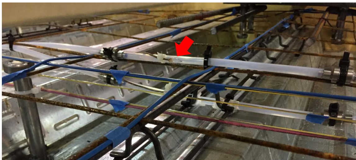
Figure 4-19 Fiber Bragg Grating sensors in CB-DA-SC with thermocouple indicated by red arrow.
