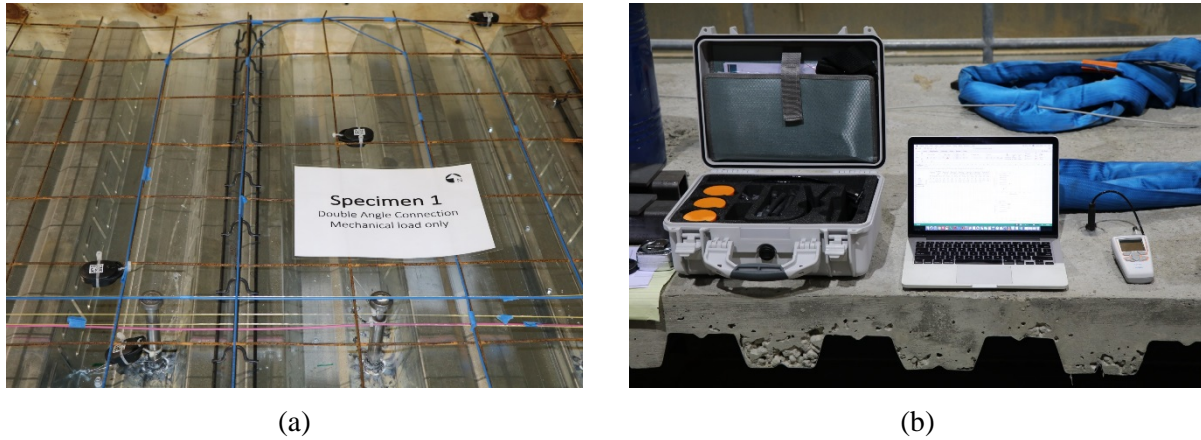
Figure 2-15 Monitoring of relative humidity in the slab during curing: (a) embedded wireless sensors (black ovals); (b) downhole relative humidity probe.
