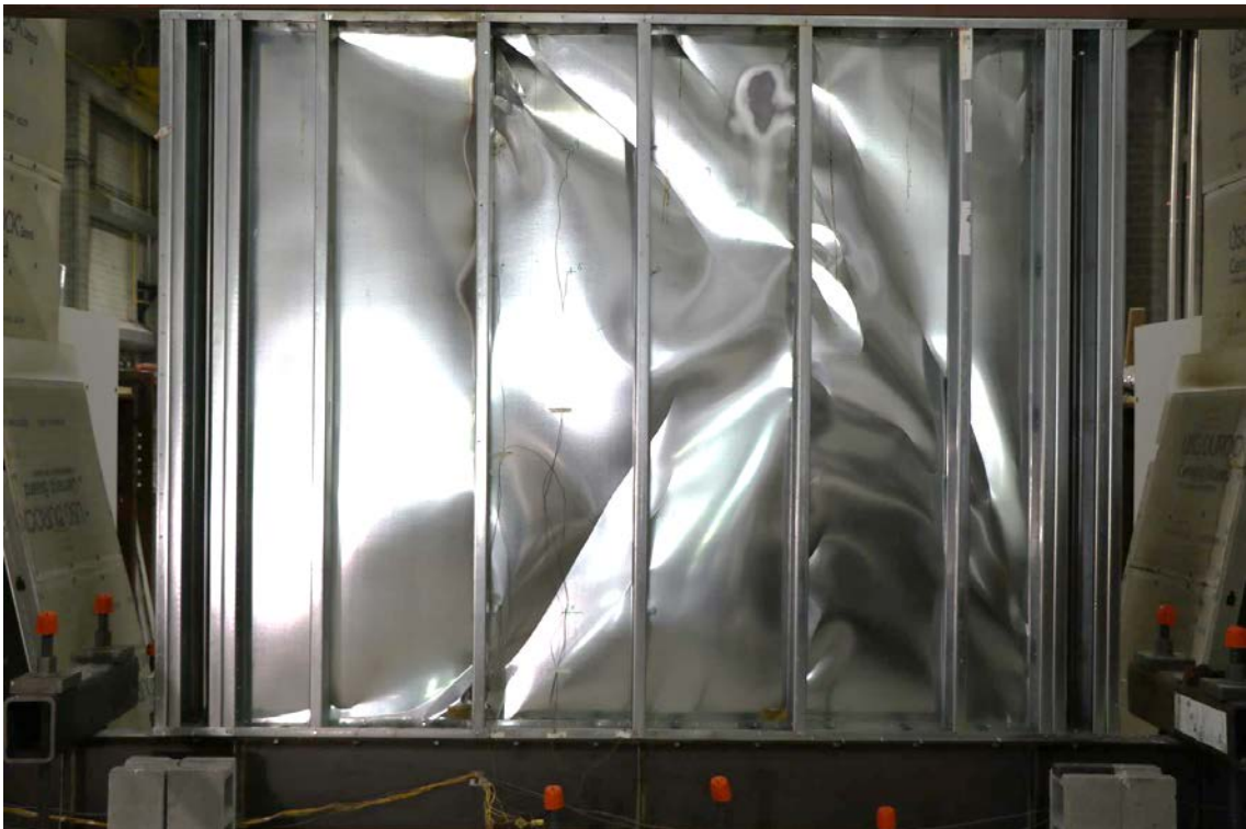
Figure 84: CFS04 – Photograph of back of metal sheathed side of the burned wall after mechanical loading to 2.8 % drift (CFS04c); nonstructural gypsum removed.
