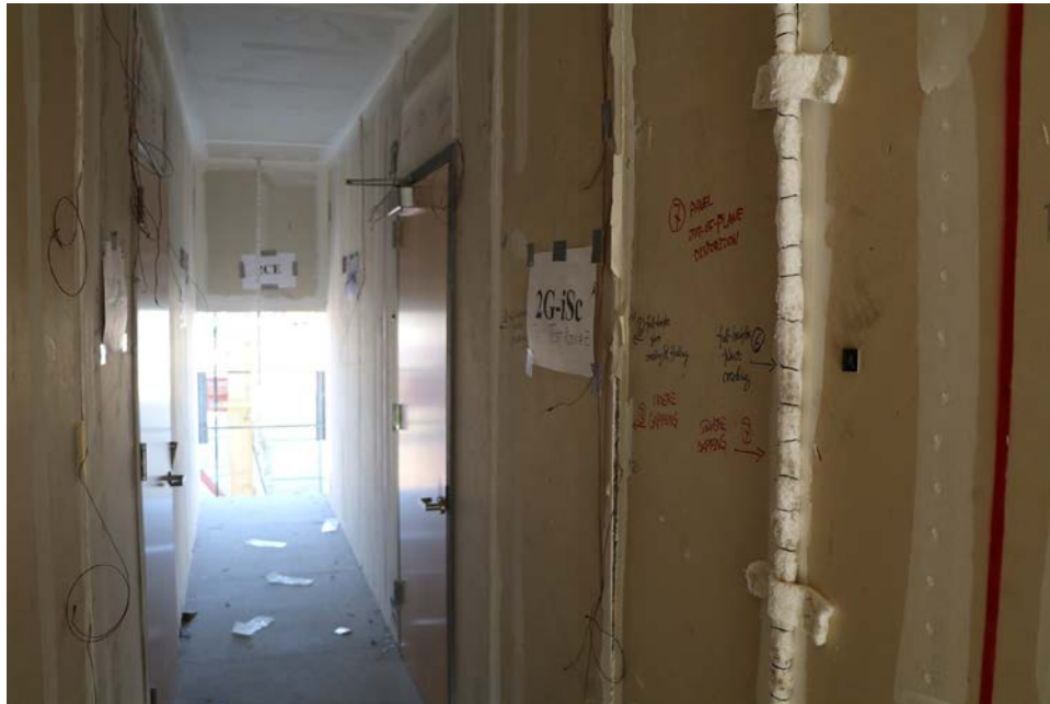
Figure 36: Photo (looking East) of 2 nd level showing opening at end of corridor in the six-story building.
