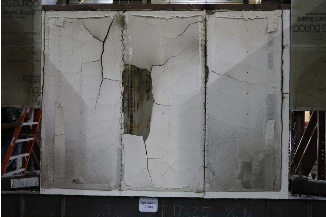
Figure 81: CFS04 – Photograph of metal sheathed side of wall after fire loading (CFS04b).
