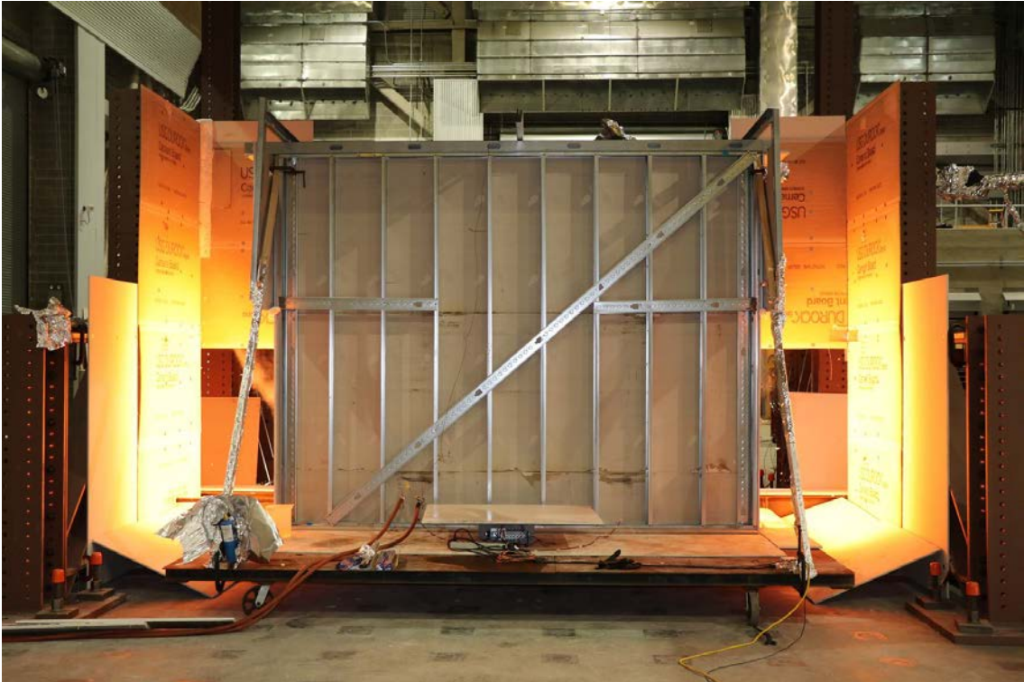
Figure 66: CFS03 - Photograph of back of compartment with redesigned fire protection for reaction frames during fire loading (CFS03b).
