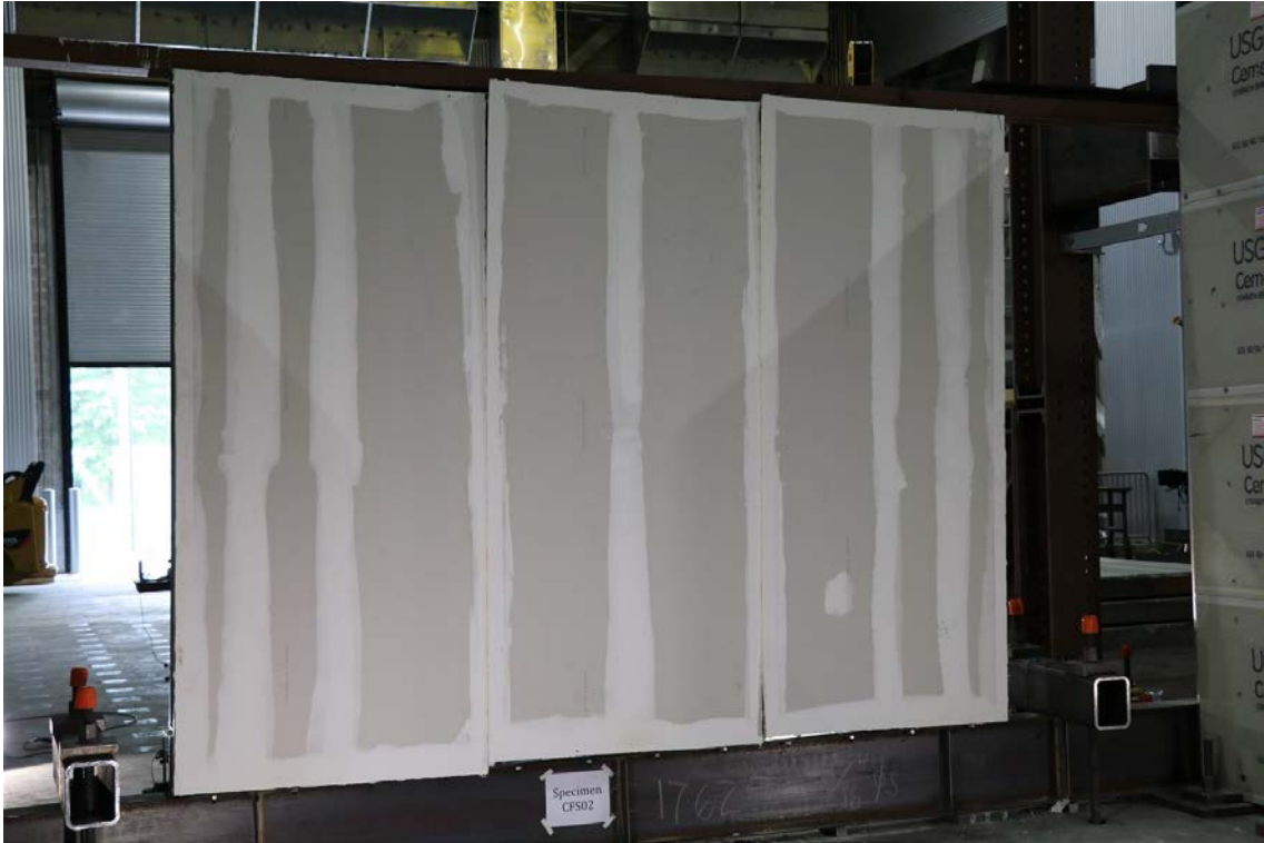
Figure 55: CFS02 - Photograph of metal sheathed side of wall after mechanical loading to 2.8 % drift (CFS02a).
