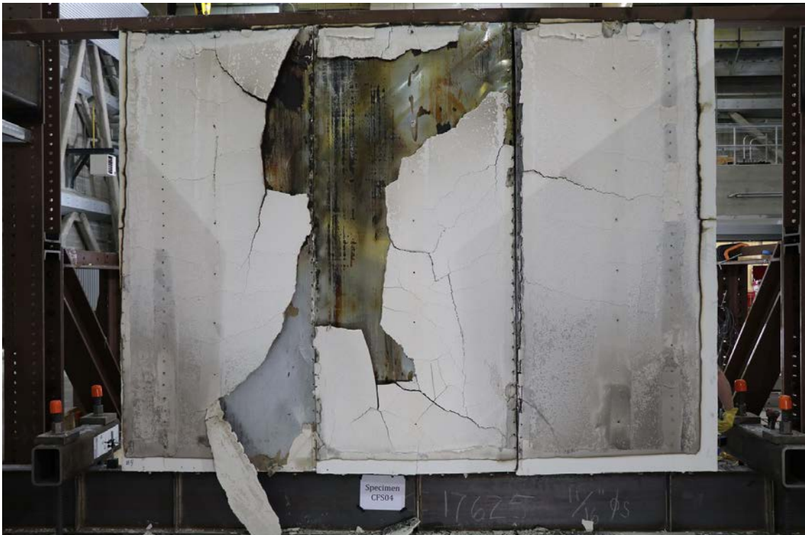
Figure 82: CFS04 – Photograph of metal sheathed side of the burned wall after mechanical loading to 2.8 % drift (CFS04c).
