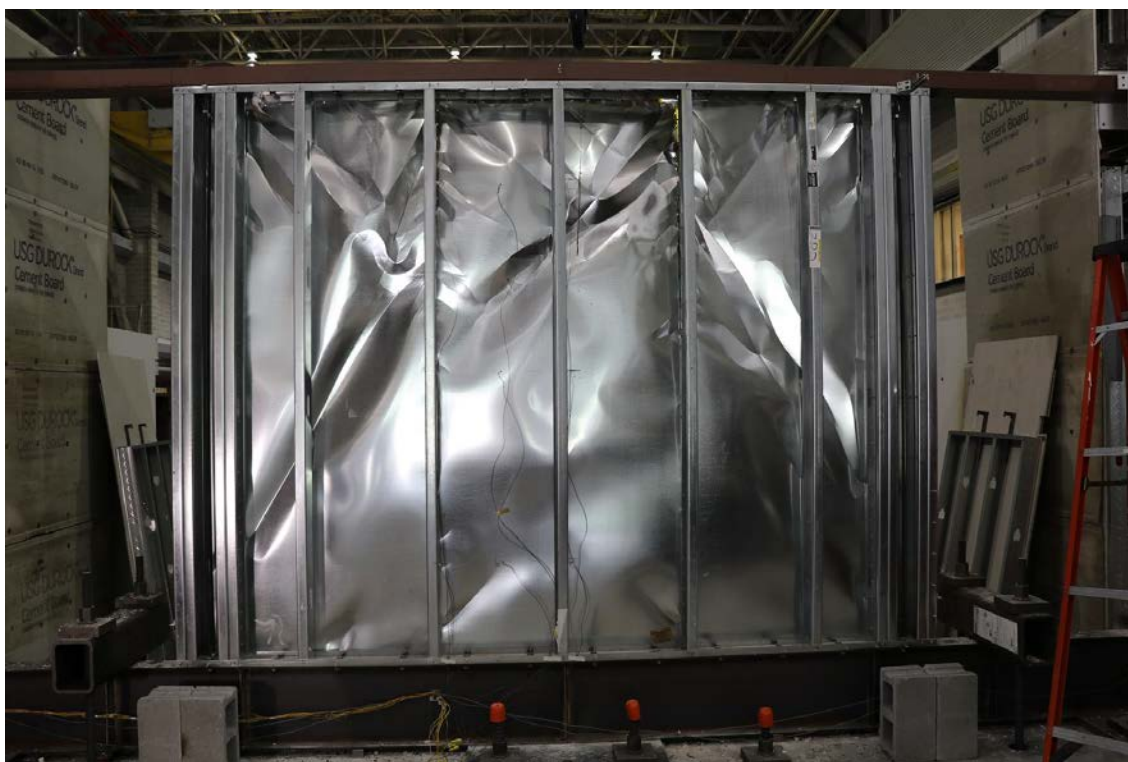
Figure 73: CFS03 – Photograph of back of metal sheathed side of the burned wall after mechanical loading to 2.8 % drift (CFS03c); nonstructural gypsum removed
