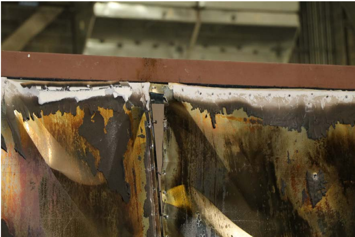
Figure 69: CFS03 – Photograph of metal sheathed side of the burned wall after mechanical loading to 2.8 % drift (CFS03c) highlighting tearing of sheet metal.
