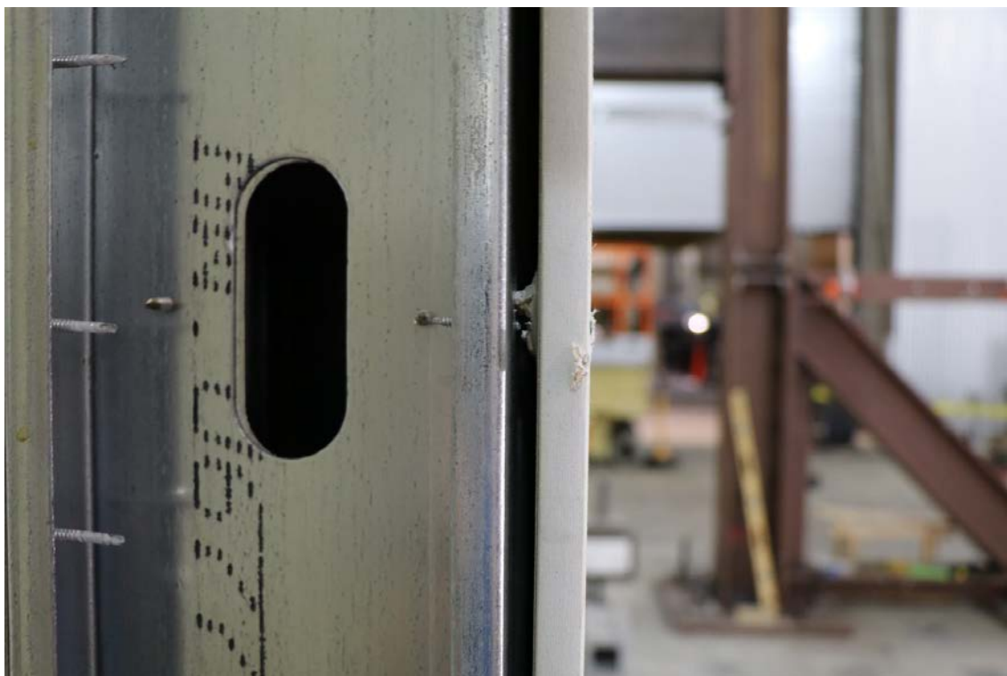
Figure 71: CFS03 – Photograph of gypsum sheathed side of wall after mechanical loading to 2.8 % drift (CFS03c) highlighting screw shearing.
