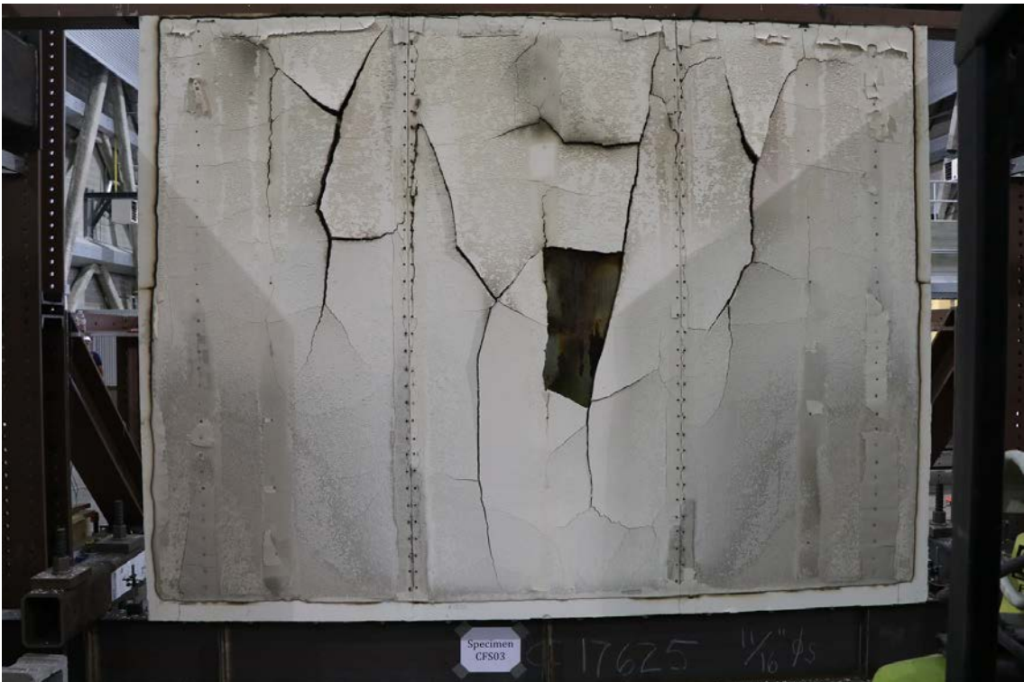
Figure 67: CFS03 – Photograph of metal sheathed side of wall after fire loading (CFS03b).
