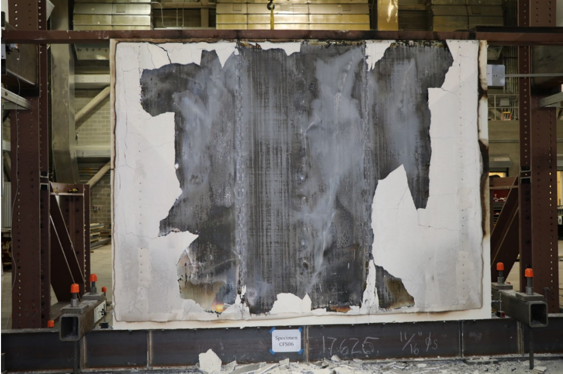
Figure 102: CFS06 – Photograph of metal sheathed side of the burned wall after mechanical loading to 2.8 % drift (CFS06c).
