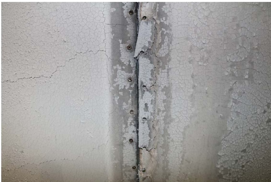
Figure 51: CFS01 - Photograph of joint detail of metal sheathed side of wall after fire loading (CFS01b).
