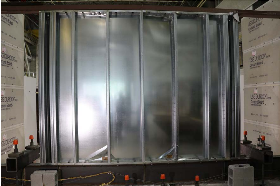
Figure 57: CFS02 - Photograph of back of metal sheathed side of wall after mechanical loading to 2.8 % drift (CFS02a); nonstructural gypsum removed.
