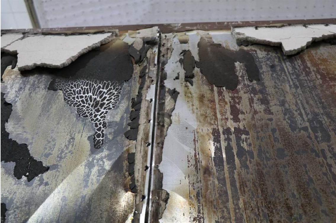
Figure 93: CFS05 – Photograph of metal sheathed side of the burned wall after mechanical loading to 2.8 % drift (CFS05b) highlighting sheeting damage.
