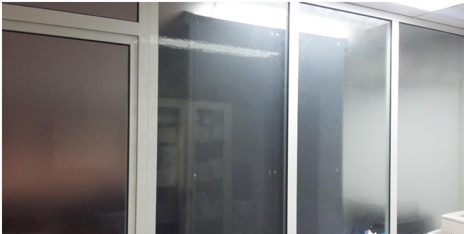
a) Core in server room.
