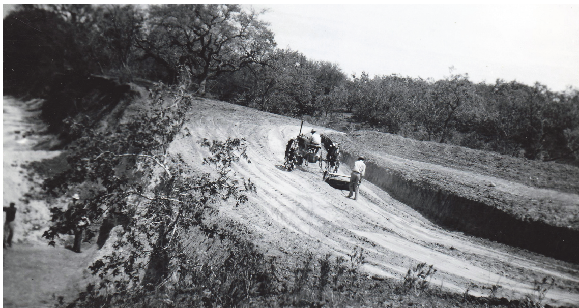
FIGURE 2. Removing overburden from Site 1, Buckner Ranch, April 1939 (41BE2-94). The tractor and Fresno scraper were hired from a local rancher who was paid $0.60/hour rental fees and $0.30/hour to drive.
