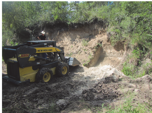
FIGURE 14. Excavation in Berclair Terrace sediments with top of the Goliad Formation evidenced by light gray sediments to the right of the small excavator.
