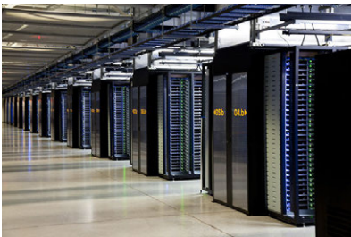
FIGURE 7.9 — Data center FACEBOOK.
