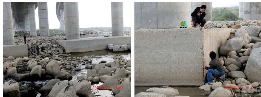
Figure 2. Photos at Da-Chia Bridge on National Highway No. 3 facing harsh environments with large-sized sediments.
