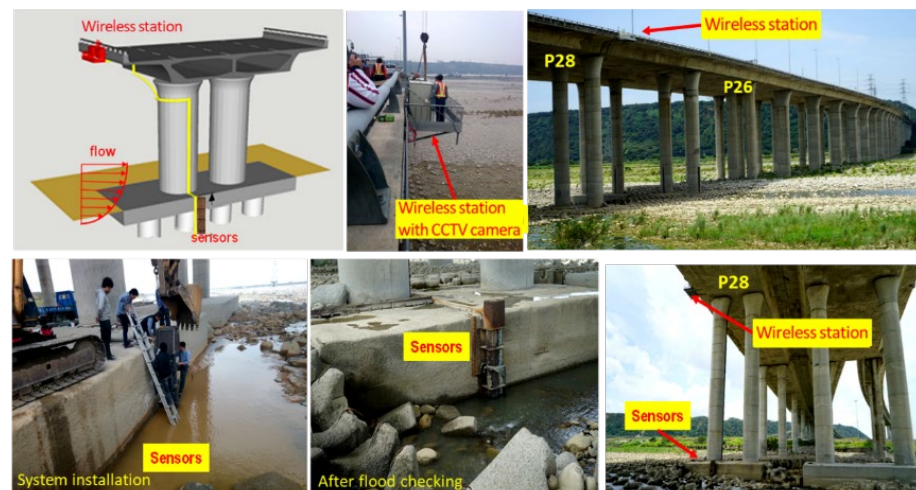
Figure 6. Installation of the scour monitoring system and the wireless station at P28 of the Da-Chia Bridge.
