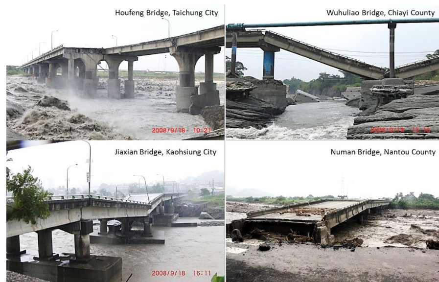
Figure 1. Bridge failure cases occurred during floods in Typhoon Sinlaku (2008).
