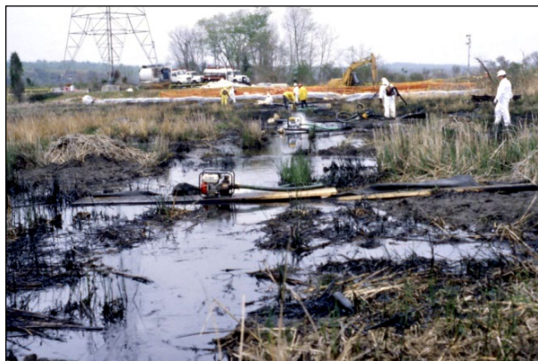
Figure 3-10. Intensive flushing operations along one of the trenches excavated at the Chalk Point, Maryland spill in April 2000. Flushing of oil from the marsh interior is very difficult. Photo credit: Jacqueline Michel.
