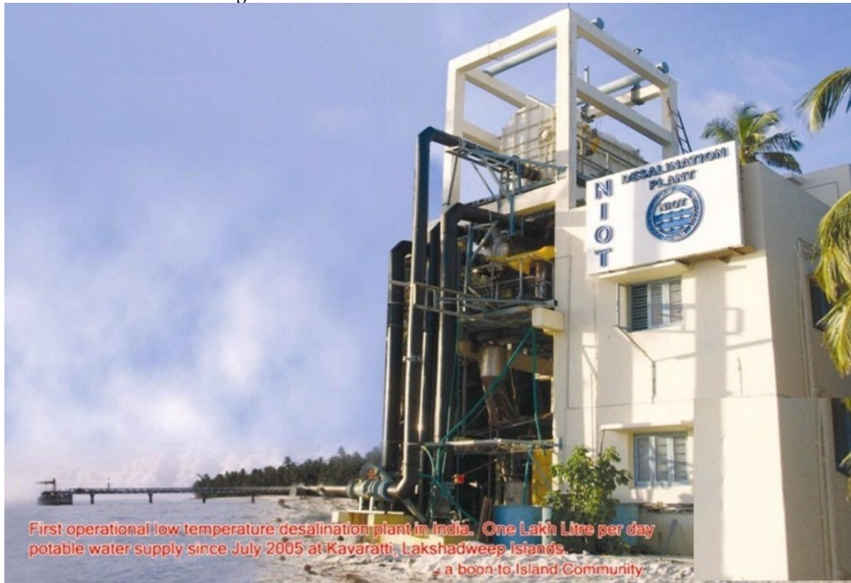
Figure 3.3: A View of the Kavaratti Desalination Plant
