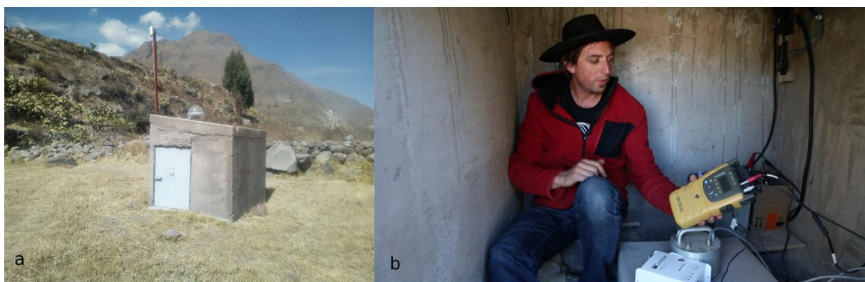
Supplementary Figure 2 | a, Picture of the hut containing the GPS and the seismic station. The antenna of the GPS is visible on the top of the hut. b, interior of the hut, with the GPS and the seismometer installation displayed.
