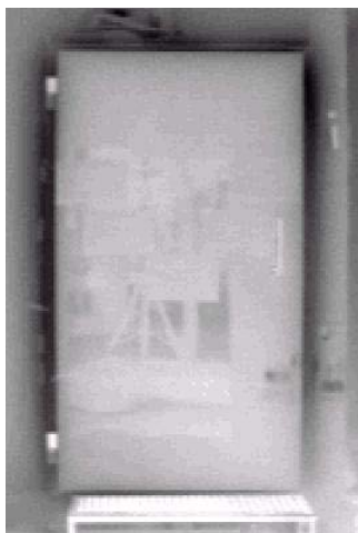
Fig. 6 Infrared picture of the cell door, taken when temperature in the cell was 20 K higher than in the guarded zone, shows thermal bridges at the door frame.
