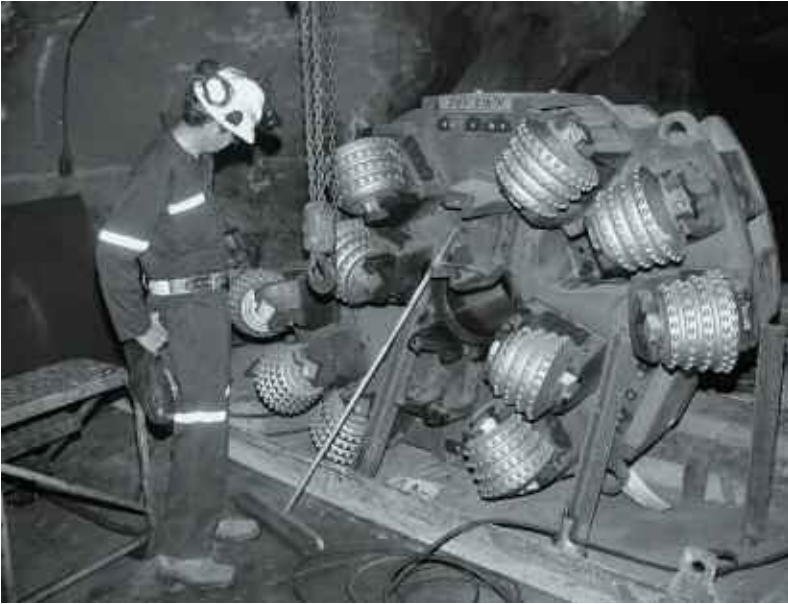
A tunnel boring machine used to excavate the new SNOLab facility in the Creighton mine. ion text caption text
