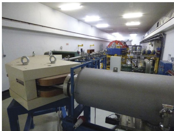
Figure 1. 6 MV Tandem accelerator (background) and the new bending magnet followed by the electrostatic analyzer of the AMS facility (foreground).
