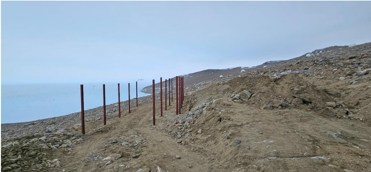
Ongoing groundwork for ICO showing the poles for the ICO containers. Photo: Simen Rykkje, Norwegian Polar Institute
