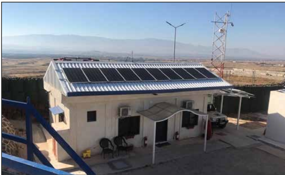
UNTSO OGG's OP56 fitted with a new array of solar panels.
