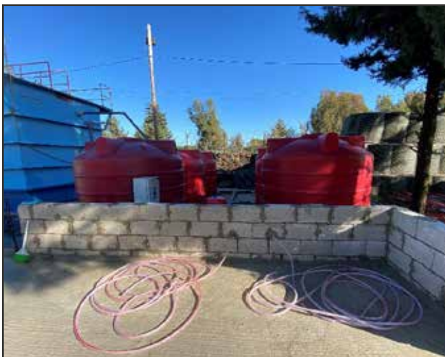
Car wash facility in Camp Faouar
