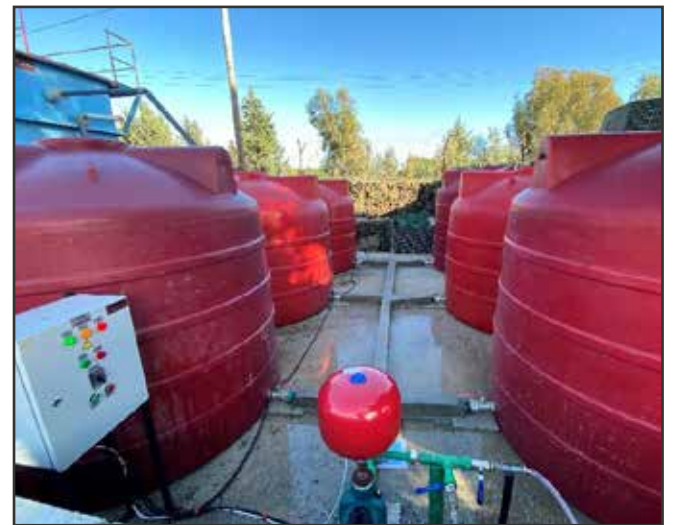
Car wash water storage tanks in Camp Faouar
