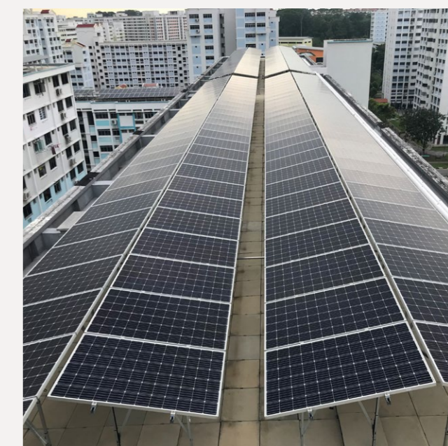
Solar panels deployed on Housing & Development Board (HDB) roofs as part of the SolarNova Programme
