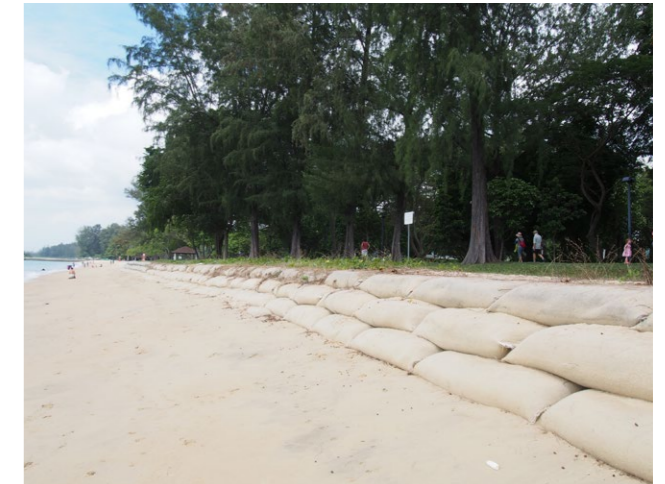
Geo-bags at East Coast Park. The geo-bags, which blend in with the beach environment, are used to prevent beach erosion while still allowing for public access.
