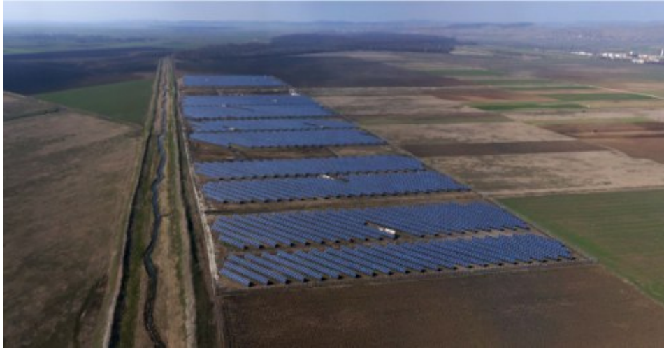
(a) Vanju-Mare PV plant image [27]
