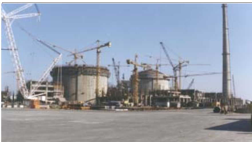
Tarapur Atomic Power Project-3&4 (2x540 MWe)
