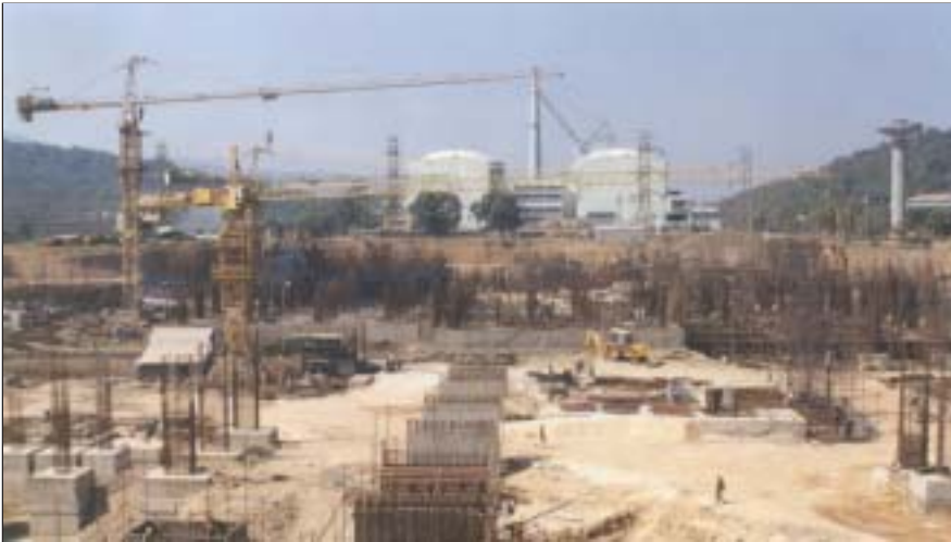
Kaiga Atomic Power Project -3&4 (2x220 MWe)
