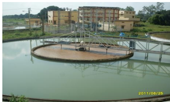
Figure 4:-Flocculator clarifiers at Lalpur (Jabalpur) water treatment plant
