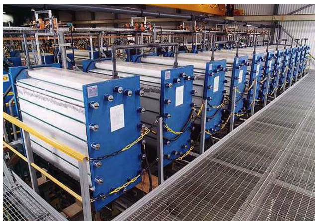
Fig. 7. Interior view of Innogy's 12 MW Regenesys™ plant at Little Barford in the UK. Figure was reproduced with kind permission from the Department for Business, Innovation and Skills, Government of U.K. and the ECS [2].
