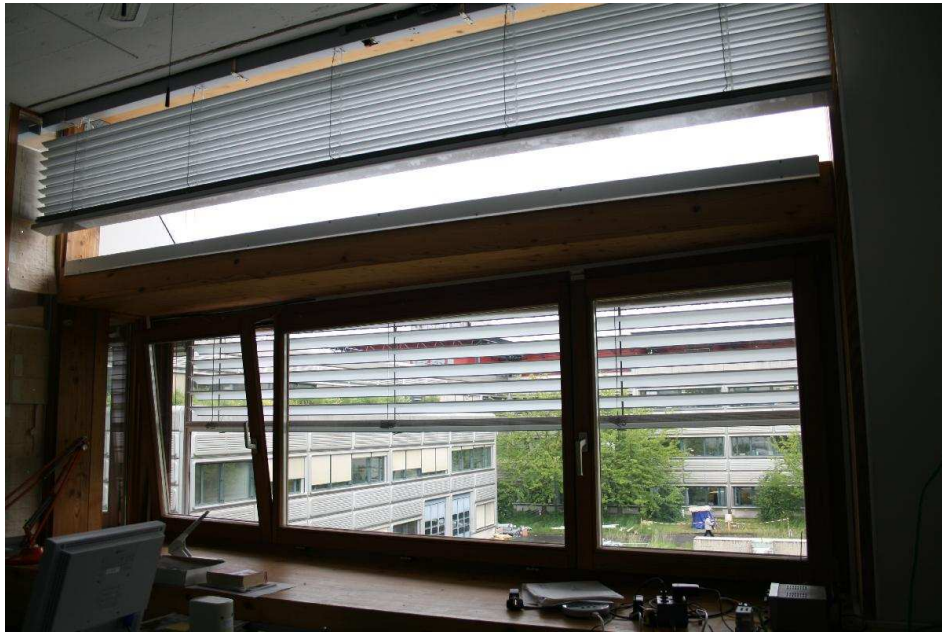
Figure 3.5: The blinds equipping office room 202. The upper indoor blinds are Baumann-Hüppe type “Genius 50”, the lower outdoor blinds are Baumann-Hüppe type “Noval 90”.
