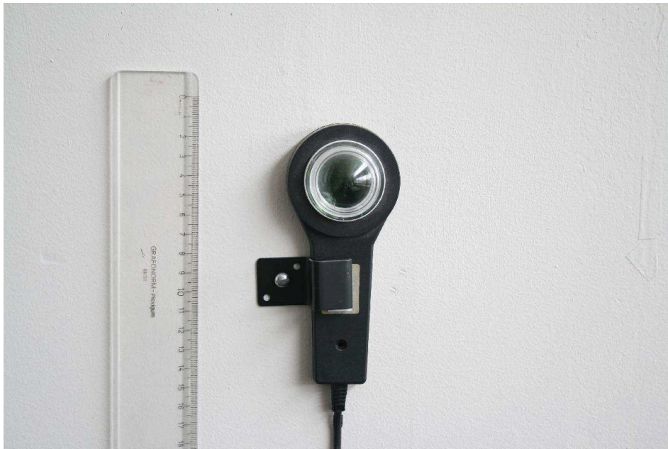
Figure 3.9: Wall-mounted illuminance sensor EB3 in office 202.
