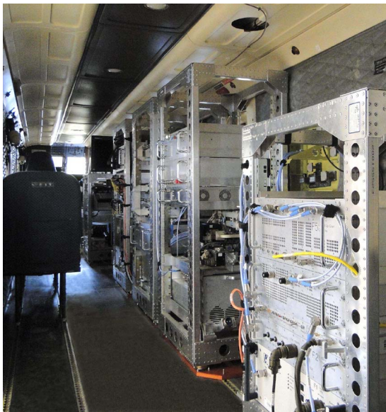
Fig. 1. The F-SAR instrument in the cabin of the Do228 aircraft. Standard instrumentation racks house the radar's electronic units.
