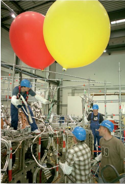
Fig. 5 Final installation of bus bars on Module 3 of the Stellarator Wendelstein 7-X.
