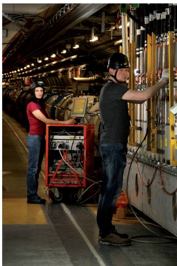
Fig. 17 ELQA measurements in the LHC tunnel.
