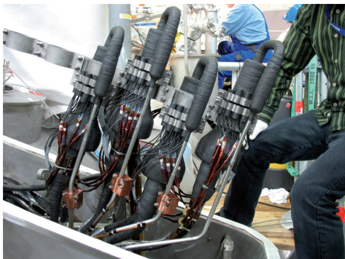
Fig. 8 Finished joints with QD boxes of non planar coils on the MSP 5-1 segment of the Stellarator Wendelstein 7-X.
