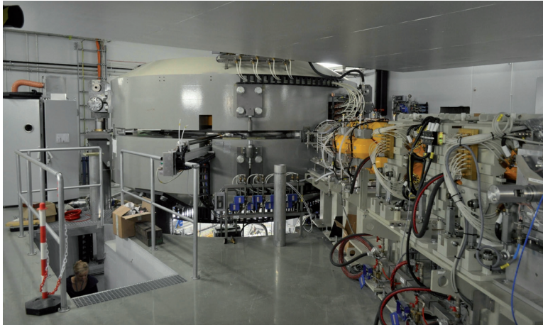
Fig. 2 The Proteus C-235 cyclotron installed at the IFJ PAN. A part of the energy degrader and selector is also visible.
