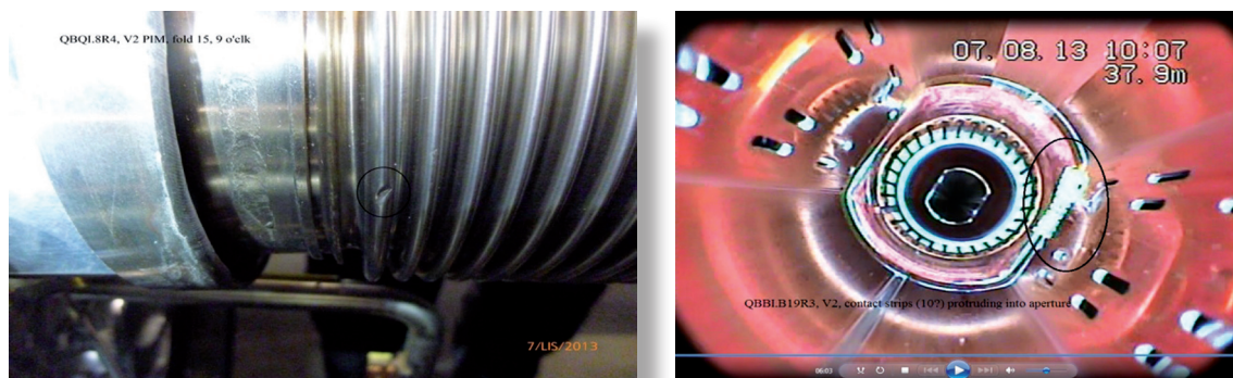
Fig. 22 Examples of mechanical damage to the Plug-in-modules resulting in their exchange: deformed beam line bellows (left) and electrical contact strips protruding into the aperture (right).
