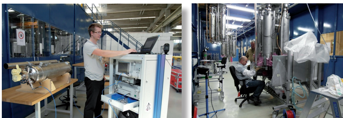
Fig. 14 Superconducting cavities in the preparation area of the AMTF hall (left); connection of cavity vacuum pipes to the insert in clean room conditions in the AMTF hall (right).
