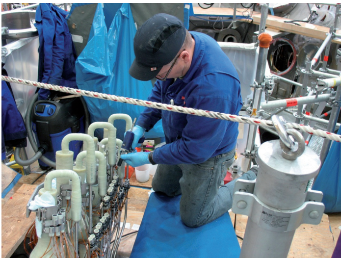
Fig. 7 Insulation of QD boxes of the Stellarator Wendelstein 7-X.
