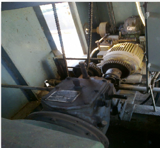
Fig.1 Local manually control of canal gate (Now a days)
