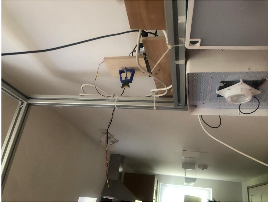
Figure 60: New Location of mmWave Antenna
