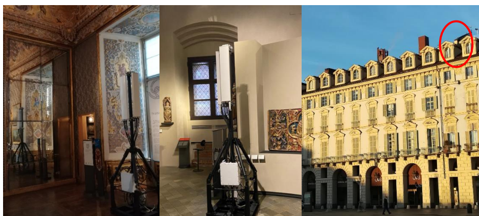
Figure 7-2: Installation for 5G indoor coverage in Sala Quattro Stagioni and Sala Acaja and rooftop antenna for the 5G outdoor coverage
