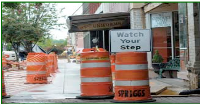
Figure 6. Sidewalk detour or construction obstacle
