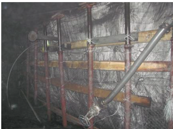
FIGURE 8: The mold bag hung on the roof.
