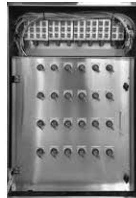
Fiber Control Panel with Internal View
