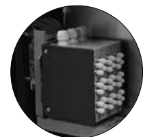
Fiber Patch Panel
