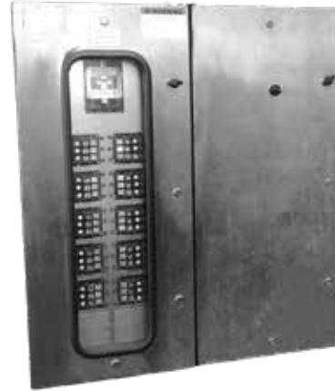
RQL Panelboard and Contactor with Main Breaker, Window, and Door Padlocking.
