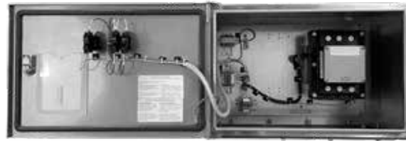
Internal View of 3-Pole RL Lighting Contactor.
