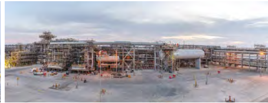
▲ Hawiyah Gas Plant Saudi Arabia
