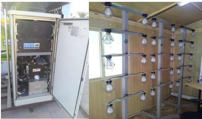
Figure 1: The ElectraGen™ PEMFC system and the 3 kW Load.
