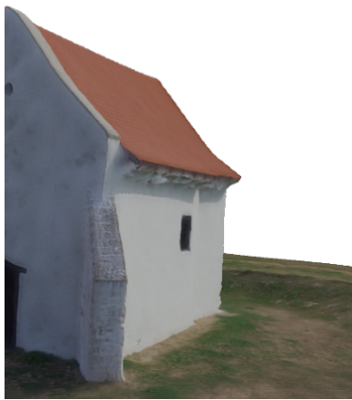
Figure 3: Part of the reconstructed chapel under the eaves full of serious flaws.
