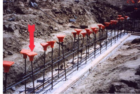
Rebar caps for impalement hazard protection
