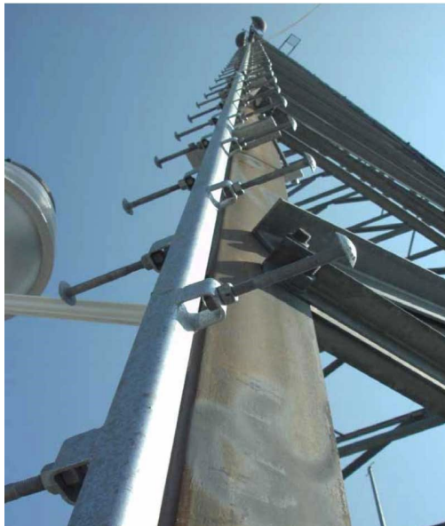
Step bolts on tower Tuf-Tug Products
