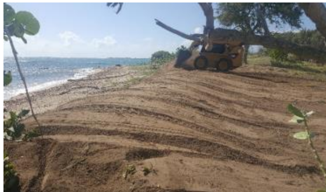
Figure 0-18: Construction of sand mounds at Playa Tamarindo (Protectores de Cuencas, used with permission)
