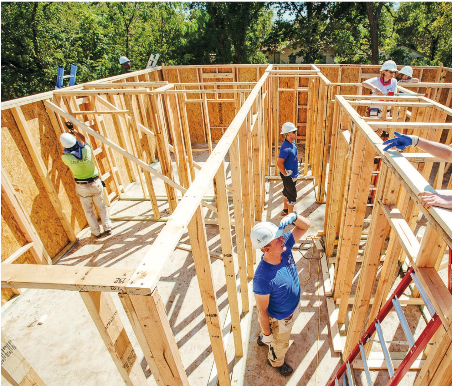
BREAKING GROUND A group of Habitat for Humanity volunteers frame a home in Fort Worth, Texas.
