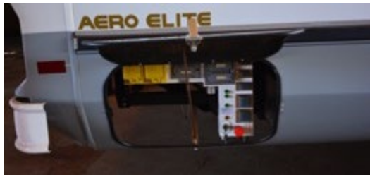
Figure 9. Bus export power unit.
