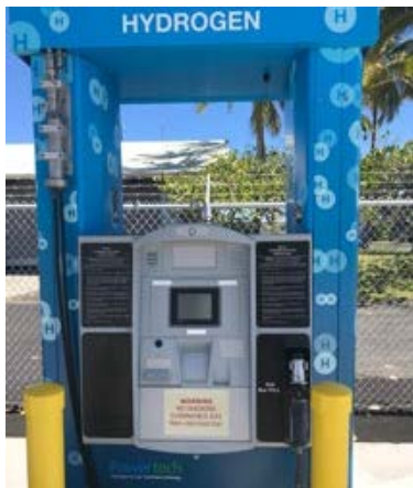
Figure 6. Hydrogen station dispenser.
