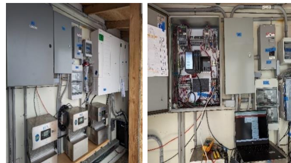
Figure 3. DC microgrid components in a dedicated electrical room (left) and system's controller box (right).
