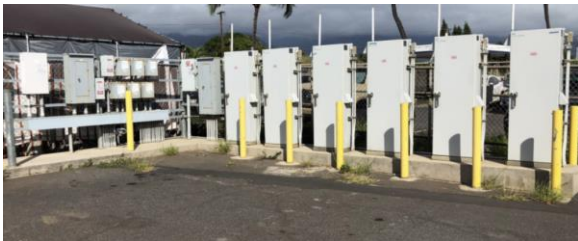
Figure 1. Sunverge SIS BESS + PV units on Maui.
