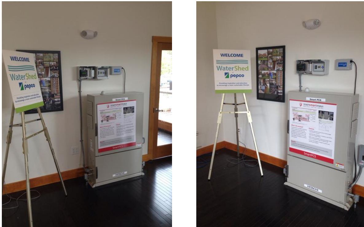
Figure 20: Hitachi inverter at Watershed Demonstration Center.
