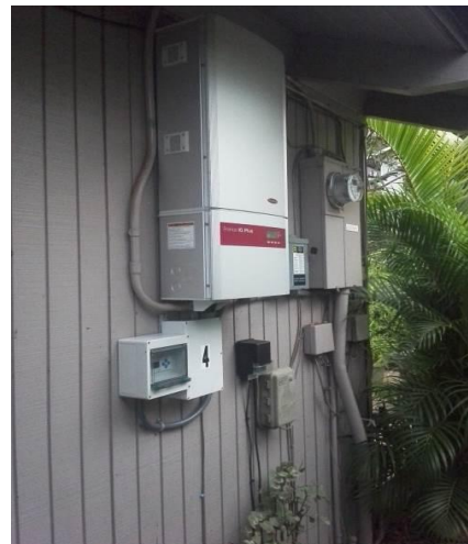
Figure 19: New advanced Fronius inverter
